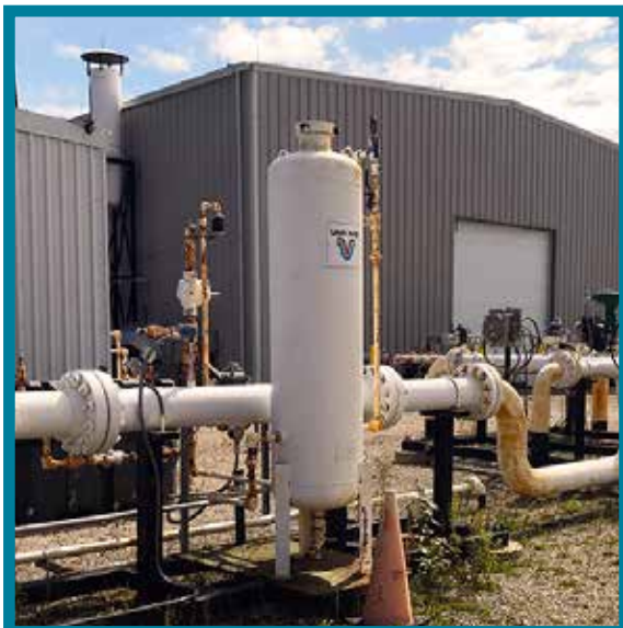
Fuel Gas Dryer for TEG unit at a NG Processing Facility.
