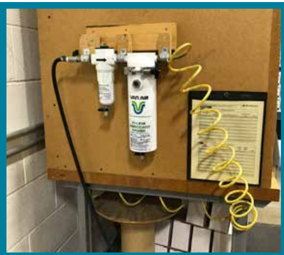
An Inline Desiccant Dryer and F200-15 filter being used on a ultrasonic welder.
